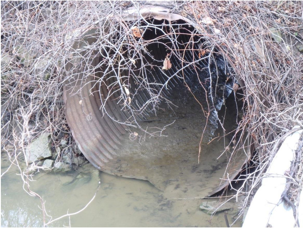
Photo 15 – Sediment Deposition in Culvert Near East Site Limit
