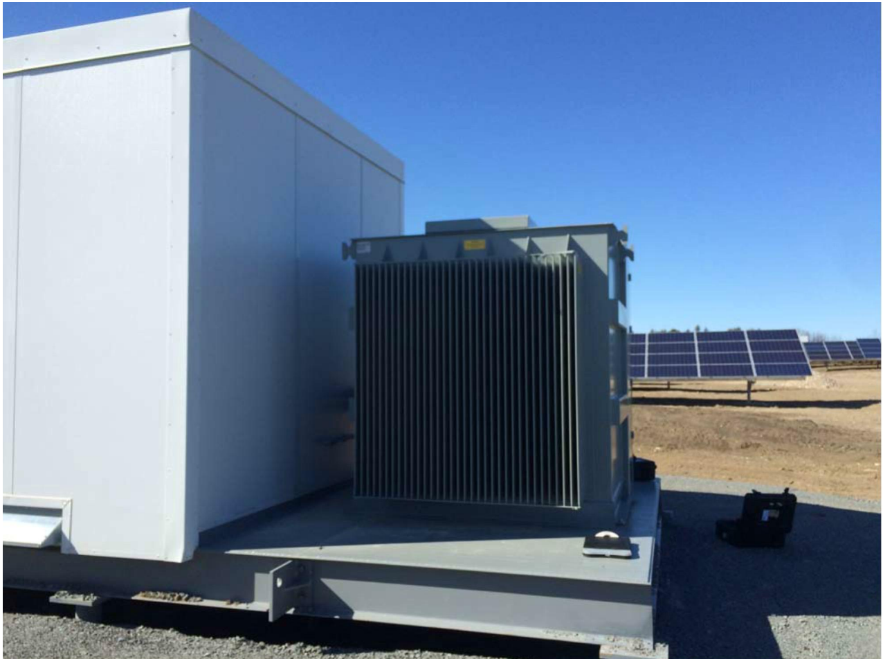
Figure 1b: 1600 kVA Transformer and Inverter Enclosure
