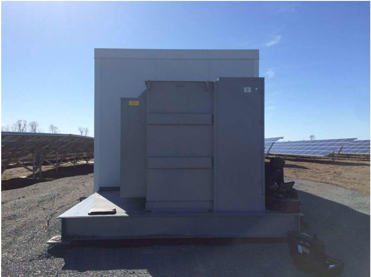
Figure 1a: 1600 kVA Transformer and Inverter Enclosure
