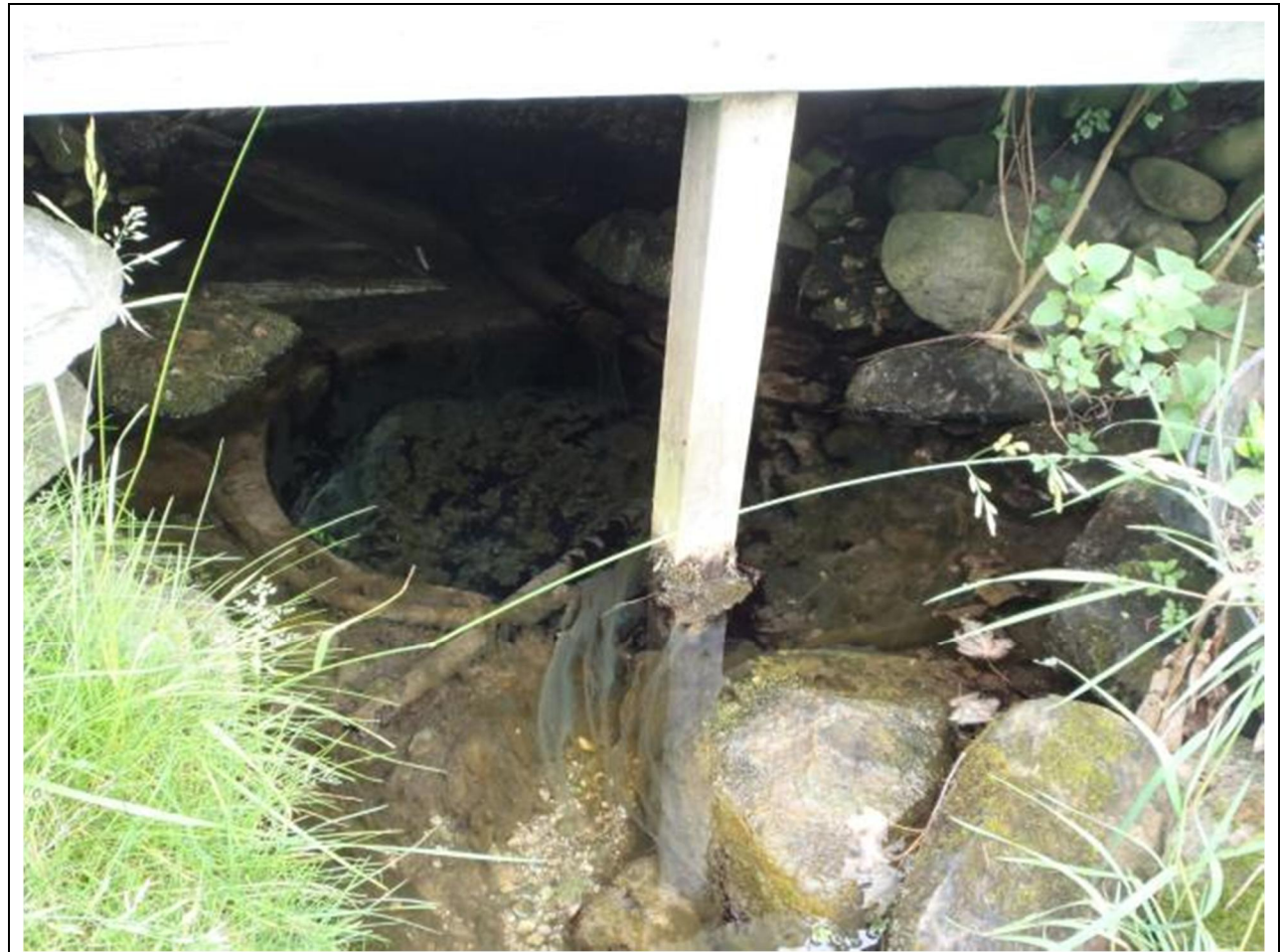
Photograph 44, facing east. Seepage Area 3 filling and over flowing from a concrete cylinder and feeding Unnamed Stream 5.
