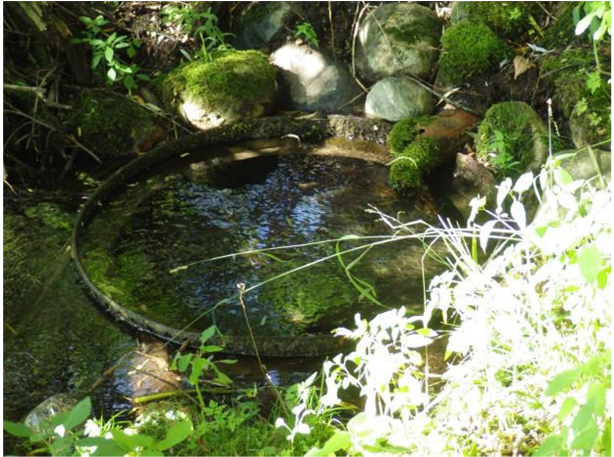
Photograph 42. Seepage Area 1 flowing from a horizontal circular steel cylinder (approximate diameter 1 m).
