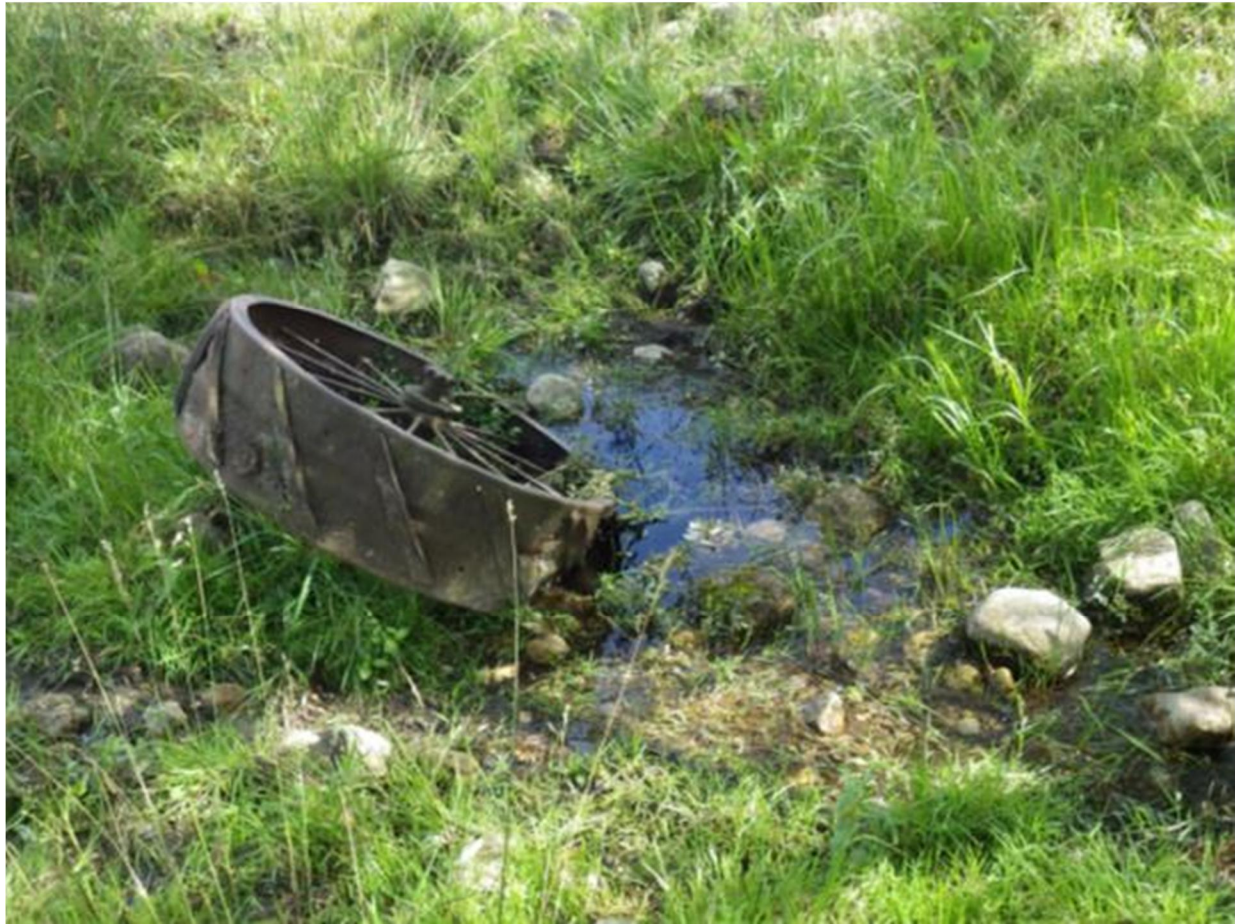
Photograph 43, facing south. Seepage Area 2 flowing from a horizontal steel cylinder (below the water surface, approximate diameter 1 m).
