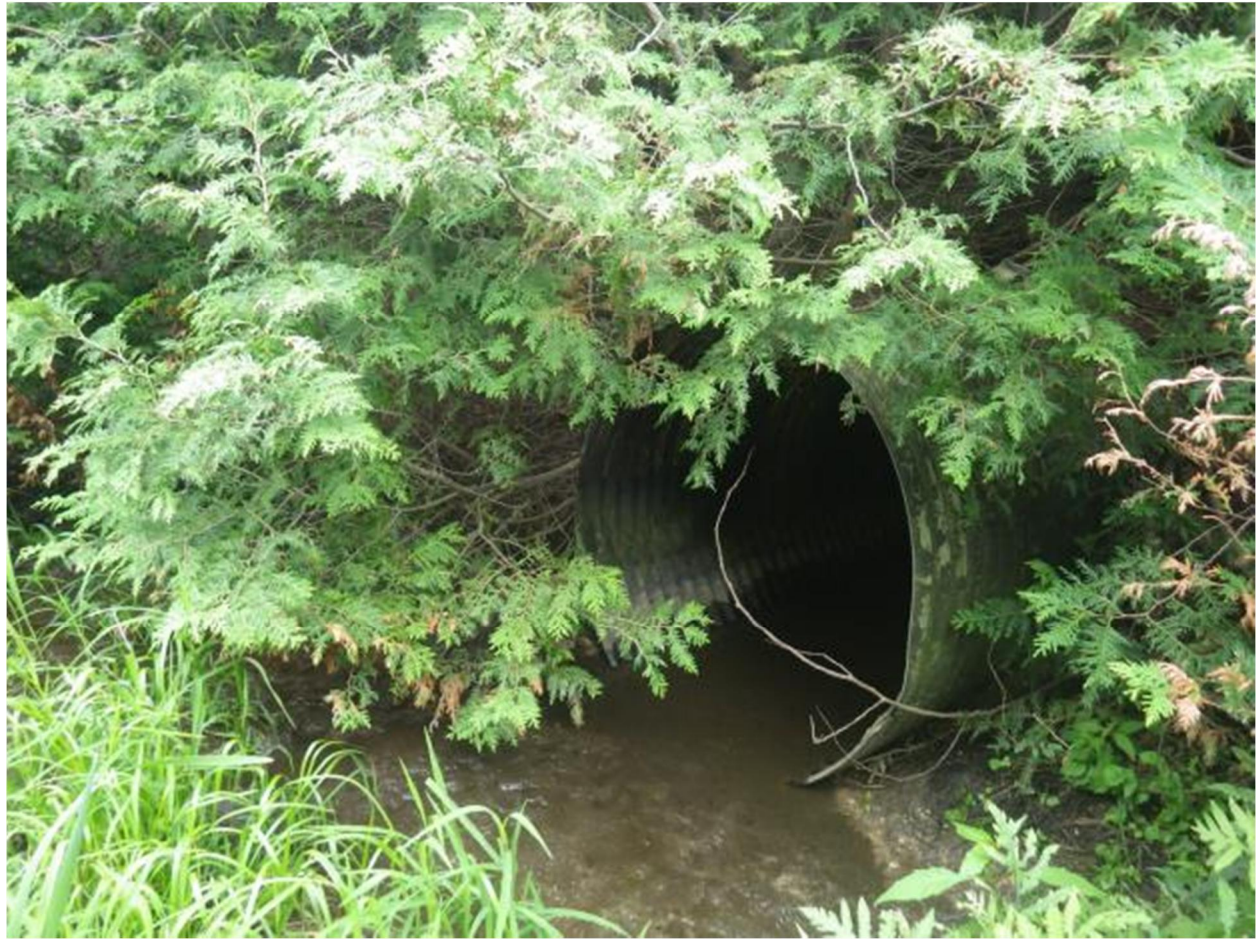
Photograph 25, facing southeast. Tributary 2 to the Beatty Saugeen River, immediately north of Grey Road 9.
