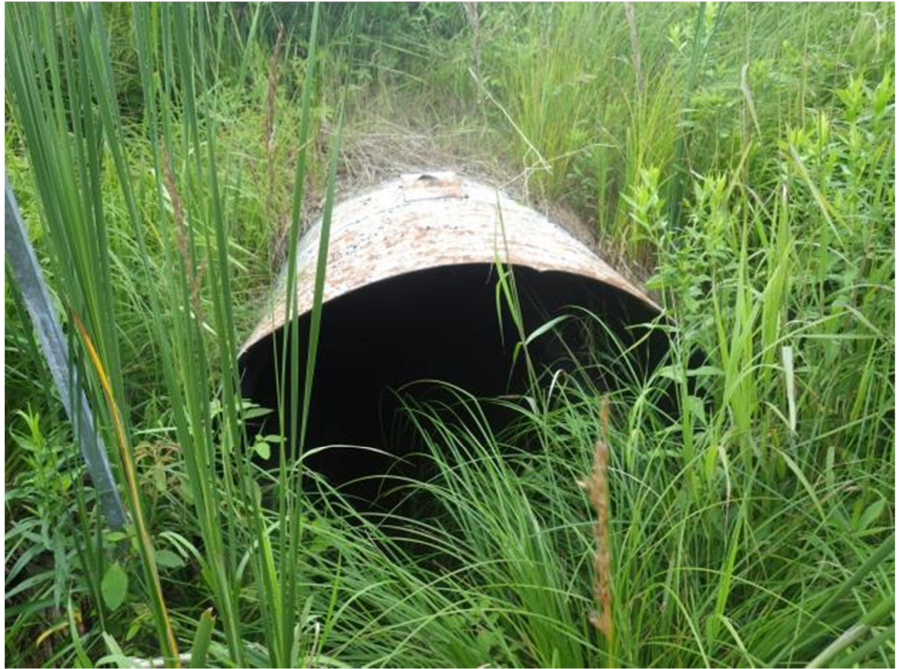
Photograph 24, facing north. Tributary 2 to the Beatty Saugeen River, flowing southward within the project location, under Grey Road 9 via a CSP culvert.
