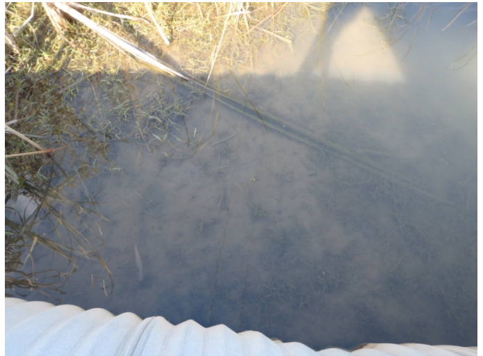
Photo 42: Lake-j (tile 10) - Looking at substrate at CSP culvert on Haldimand Road 50, approximately 300 m north of the lake shore.
