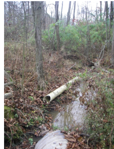
Photo 19: Lake-d (tile 15) - Looking downstream at CSP culvert and channel from ATV trail in wooded area. Site is located east of Hald-Dunn Townline Road between Rainham Road and the lakeshore.
