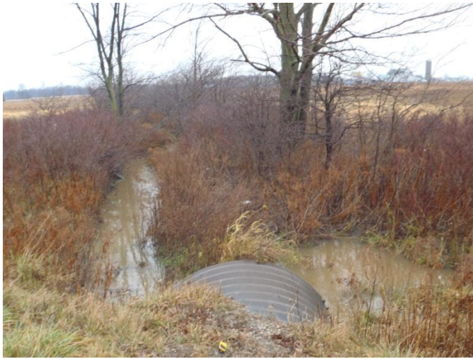
Photo 19: Hem-g (tile 4) - Looking upstream (northeast) at channel from CSP culvert. Site is located on Haldimand Road 20 between Concession 6 and Link Road.
