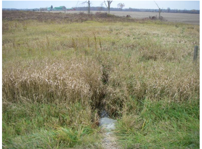
Photo 14: Hem-d (tile 4) - Looking downstream (southwest) at drain feature associated with CSP culvert flowing low-laying area. This site is on Haldimand Road 20 near the intersection with Kohler Road. The racetrack can be seen in the distance.
