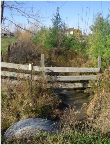
Photo 8: Evans-c (tile 12) - Looking at upstream (north) from CSP culvert flowing under Bains Road, south of Haldimand Road 20, between Haldimand Road 50 and South Cayuga Road.
