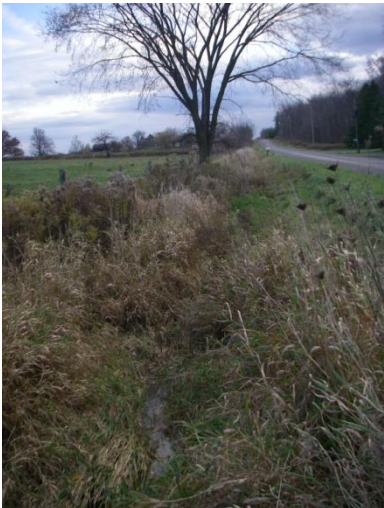
Photo 3: Evans-a (tile 9) - Looking east at roadside drain contributing to watercourse at upstream end of CSP culvert. This site is located on Bains Road between Sutor Road and Haldimand Road 50.
