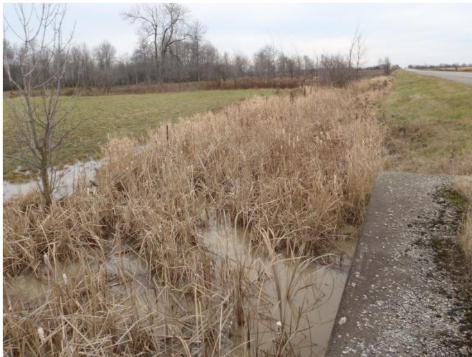
Photo 1: Ston-a (tile 19) - Looking upstream (southeast) from concrete culvert at flooded vegetation and roadside drain. Site is located on Haldimand Road 20 between Concession 10 and Concession 11 W-1.
