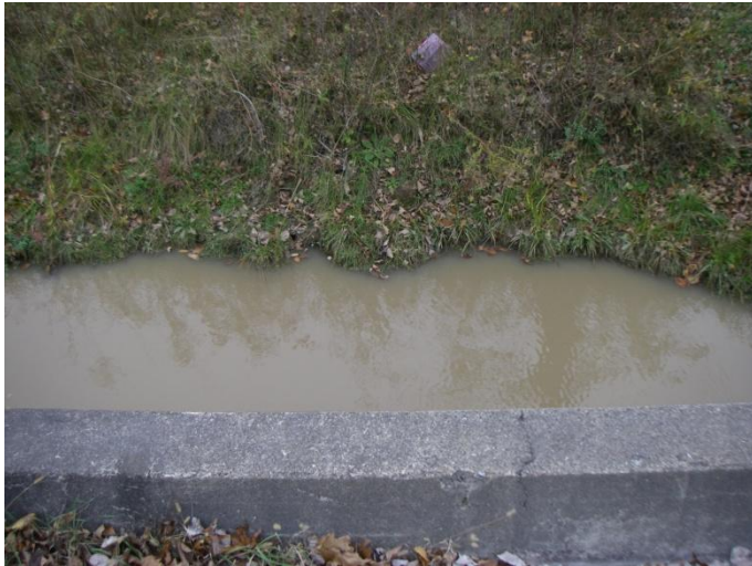
Photo 22: Ward-k (tile 9) - Looking north at upstream end of concrete culvert on watercourse. This site is located on Bains Road between Sutor Road and Haldimand Road 50.
