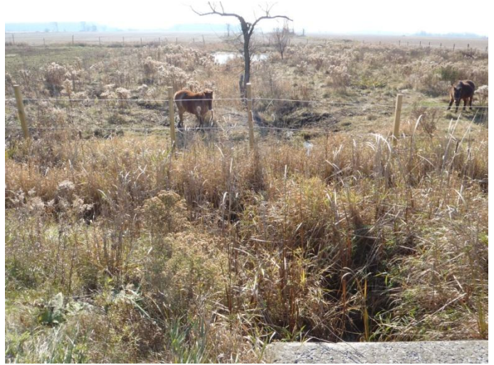
Photo 7: Ward-c (tile 8) - Looking downstream (east) at concrete culvert on south side of Haldimand Road 20, between Wilson Road and Sutor Road.
