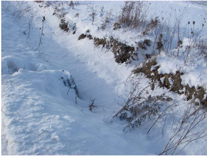
Photo 43: Hem-n (tile 6) - Looking at CSP culvert and roadside drain on north side of Concession 4. Site is located on Concession 4, between Kohler Road and Haldimand Road 20.
