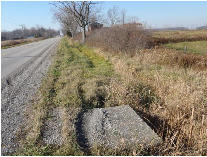
Photo 6: Ward-c (tile 8) - Looking upstream (west) at concrete culvert on north side of Haldimand Road 20, between Wilson Road and Sutor Road.
