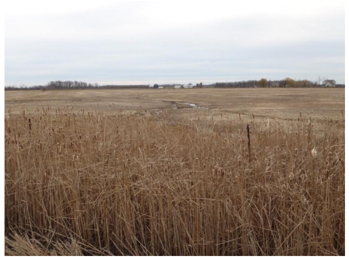
Photo 11: Ston-c (tile 18) - Looking downstream (west) from concrete culvert at cattail vegetation in roadside drain and channel flowing through agriculture field in the distance. Site is located on Haldimand Road 20 between Old Talbot Road and Haldimand Road 53.
