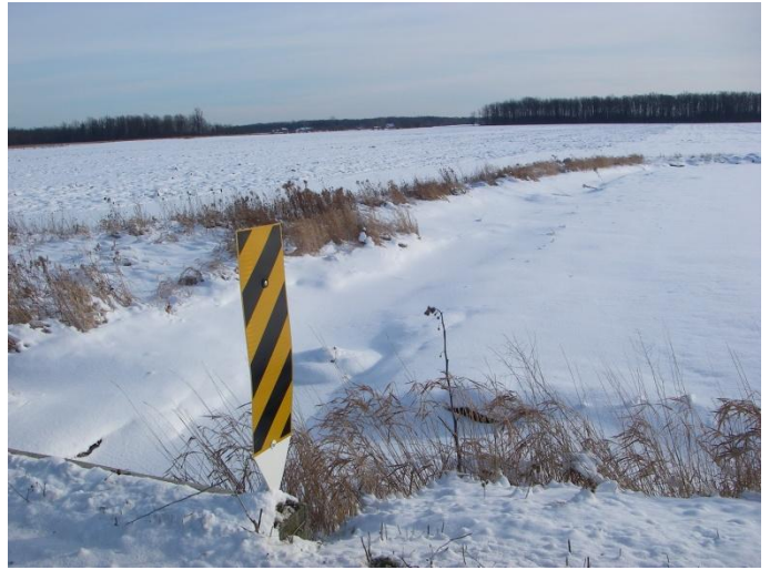
Photo 46: Hem-o (tile 6) - Looking south at outflow of concrete culvert and channel flowing through agriculture lands. Site is located on Concession 4, between Kohler Road and Haldimand Road 20
