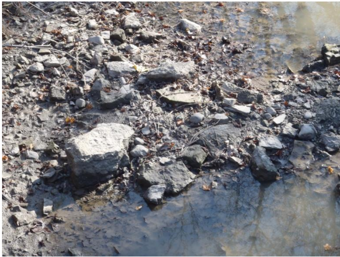
Photo 22: Evans-h (tile 10) - Looking at substrate at concrete culvert on Lakeshore Road. Site is located west of White Cap Lane and Haldimand Road 50, approximately 20 m north of the lake shore.
