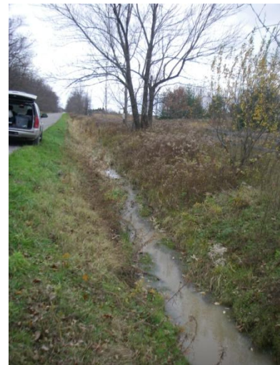
Photo 23: Ward-k (tile 9)- Looking upstream (west) of concrete culvert on north side of Bains Road. This site is located on Bains Road between Sutor Road and Haldimand Road 50.
