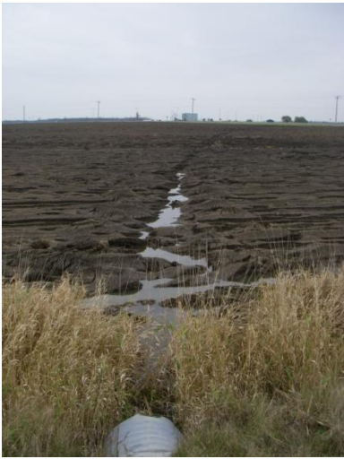
Photo 13: Hem-d (tile 4) - Looking upstream (east) at drain feature associated with CSP culvert flowing through plowed agricultural field. This site is on Haldimand Road 20 near the intersection with Kohler Road.
