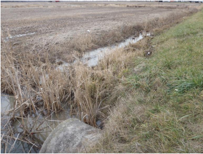
Photo 12: Ston-d (tile 18) - Looking upstream (east) from concrete culvert at agriculture field and roadside drain. Site is located on Haldimand Road 20 between Old Talbot Road and Haldimand Road 53.
