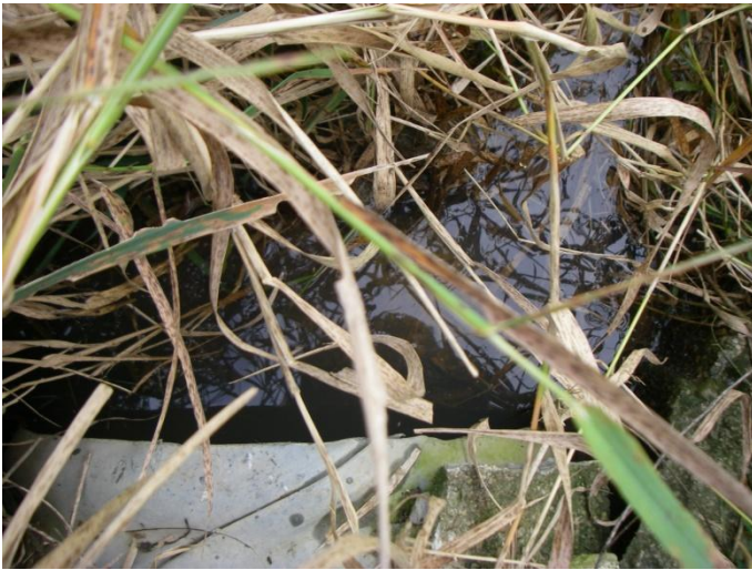
Photo 21: Ward-j (tile 8) - Substrate in drain feature at CSP culvert in a field. Site is located west of Haldimand Road 50 between Haldimand Road 20 and Bains Road.
