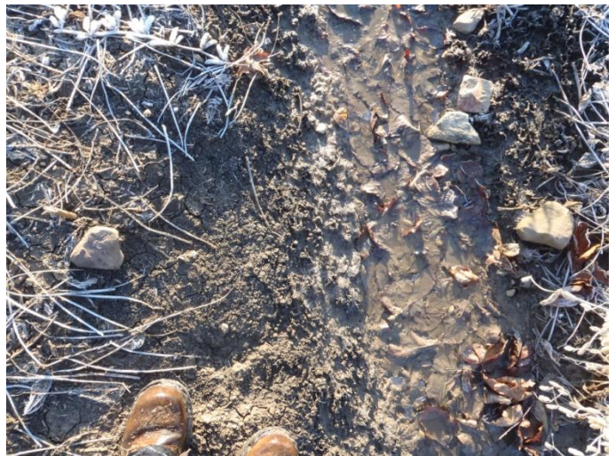
Photo 21: Evans-i (tile 11) (field data sheet 33.1) - Existing substrate conditions in channel. Site is located north of Bains Road between Haldimand Road 50 and South Cayuga Road.
