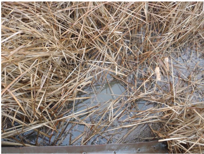
Photo 21: Hem-g (tile 4) - Existing substrate conditions at CSP culvert. Site is located on Haldimand Road 20 between Concession 6 and Link Road.
