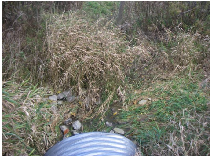
Photo 2: Evans-a (tile 9) - Looking at existing conditions at upstream end of CSP culvert. This site is located on Bains Road between Sutor Road and Haldimand Road 50.
