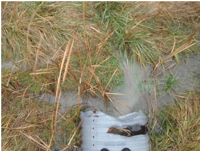
Photo 35: Hem-i (tile 3) - Existing substrate conditions at upstream end of CSP culvert. Site is located on Haldimand Road 20 between Concession 8 and Link Road.
