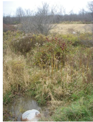
Photo 12: Hem-c (tile 4) - Looking upstream (east) at small pool and isolated drain feature associated with CSP culvert flowing through lowland vegetation, agricultural field and eventually into a woodlot. This site is on Haldimand Road 20 between Concession 5 and Concession 6.
