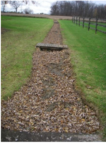
Photo 22: Hem-h (tile 4) - Looking upstream (west) from CSP culvert in laneway at linear channel flowing through a residential property. Site is located west of Haldimand Road 20, between Concession 4 and Concession 5.
