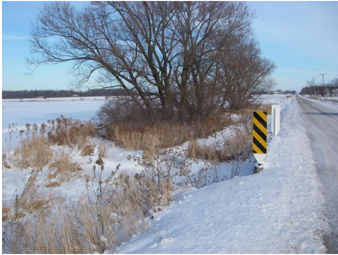
Photo 45: Hem-o (tile 6) - Looking east at upstream end of concrete culvert on north side of Concession 4. Site is located on Concession 4, between Kohler Road and Haldimand Road 20.
