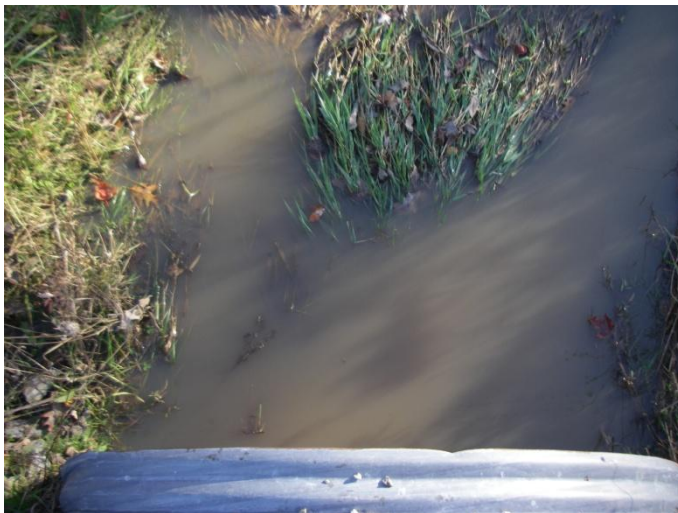
Photo 10: Evans-c (tile 12) - Looking at substrate at CSP culvert flowing under Bains Road, south of Haldimand Road 20, between Haldimand Road 50 and South Cayuga Road.
