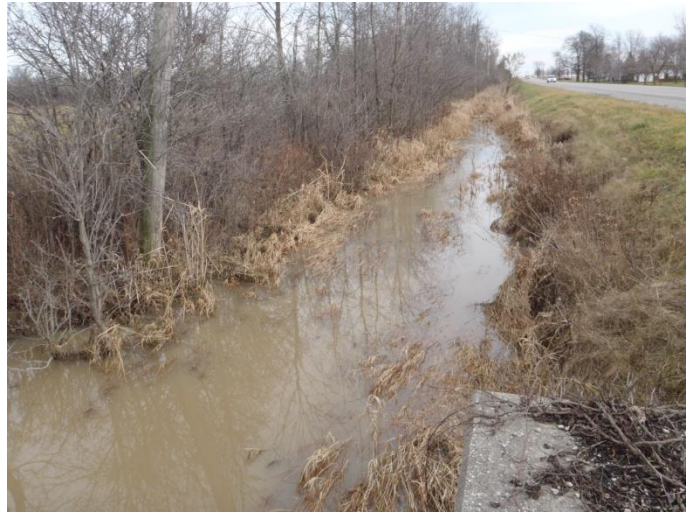
Photo 6: Ston-b (tile 19) - Looking upstream (east) from concrete culvert at flooded vegetation in roadside drain. Site is located on Haldimand Road 20 between Haldimand Road 53 and Concession 10.
