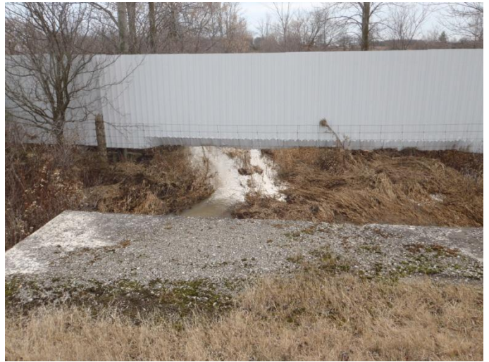
Photo 8: Ston-b (tile 19) - Looking downstream (southwest) from concrete culvert at flooded vegetation. Site is located on Haldimand Road 20 between Haldimand Road 53 and Concession 10.
