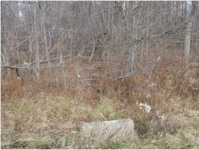
Photo 17: Ston-f (tile 18) - Looking upstream (northeast) from concrete culvert at area of channel. Site is located on Haldimand Road 20 between Dry Lake Road and Highway 3.
