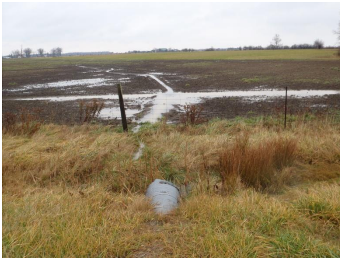
Photo 33: Hem-i (tile 3) - Looking upstream (north) at channel from CSP culvert. Site is located on Haldimand Road 20 between Concession 7 and Haldimand Road 12.
