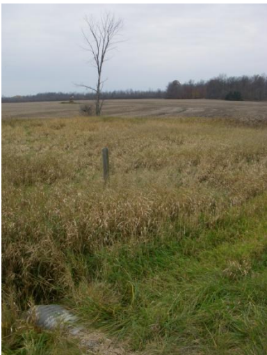
Photo 15: Hem-d (tile 4) - Looking downstream (southwest) at drain feature associated with CSP culvert flowing low-laying area (shown in previous picture) and into agricultural field (channel can be seen in the distance). This site is on Haldimand Road 20 near the intersection with Kohler Road.
