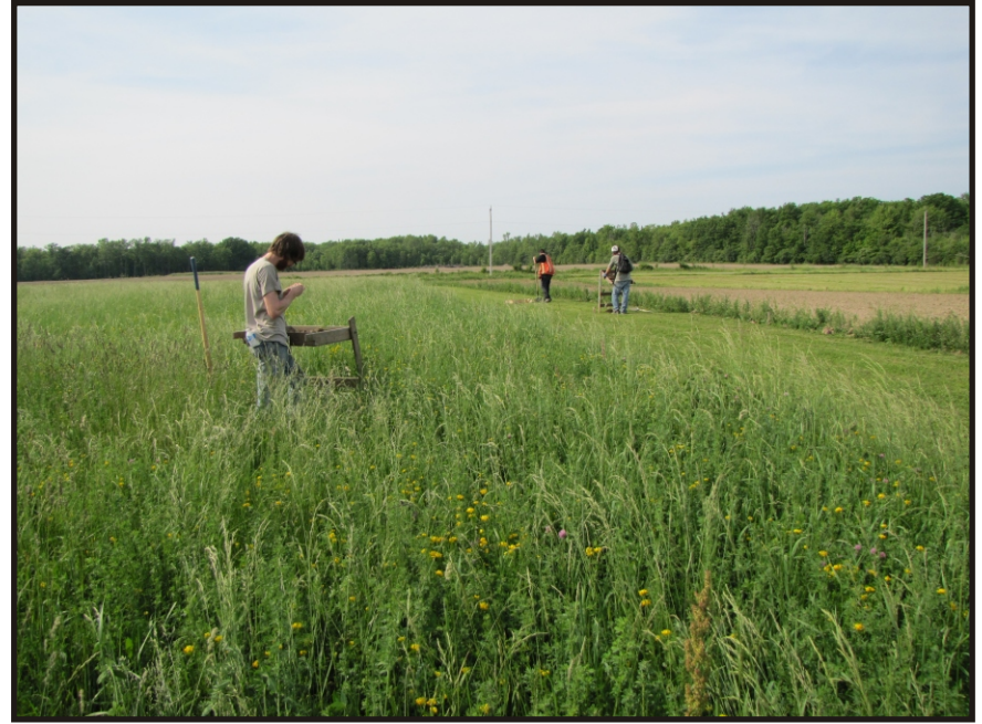
Photo 18 - Excavating Test Pits Along West Side of T23 and T26 Access Road
