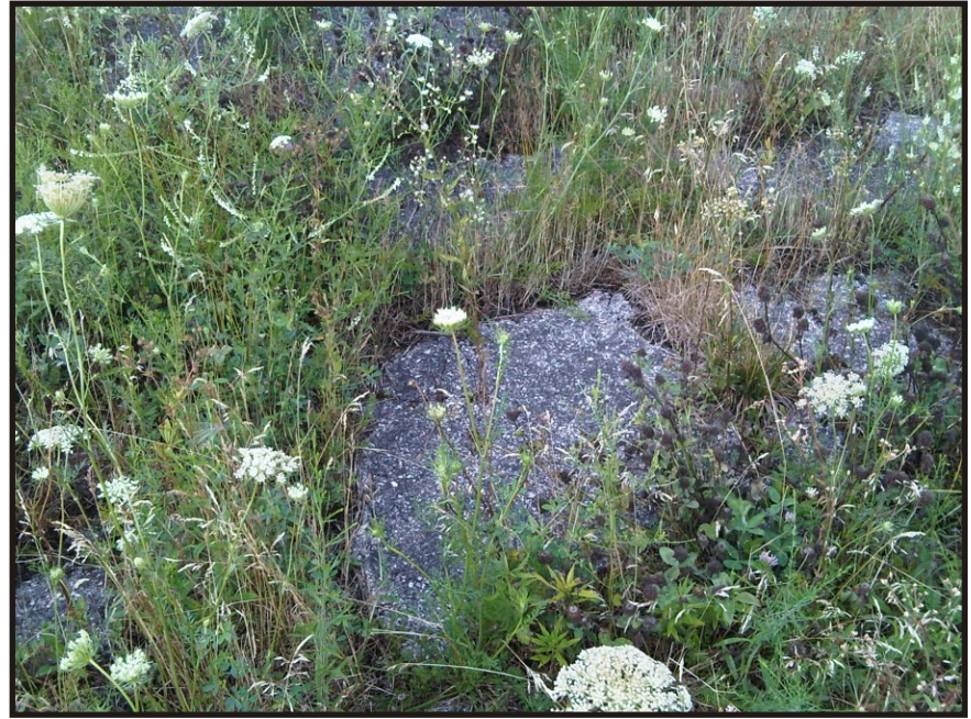
Photo 10 - Decaying Asphalt of Old Runway Under Weeds, South of Access Road for Turbine 61
