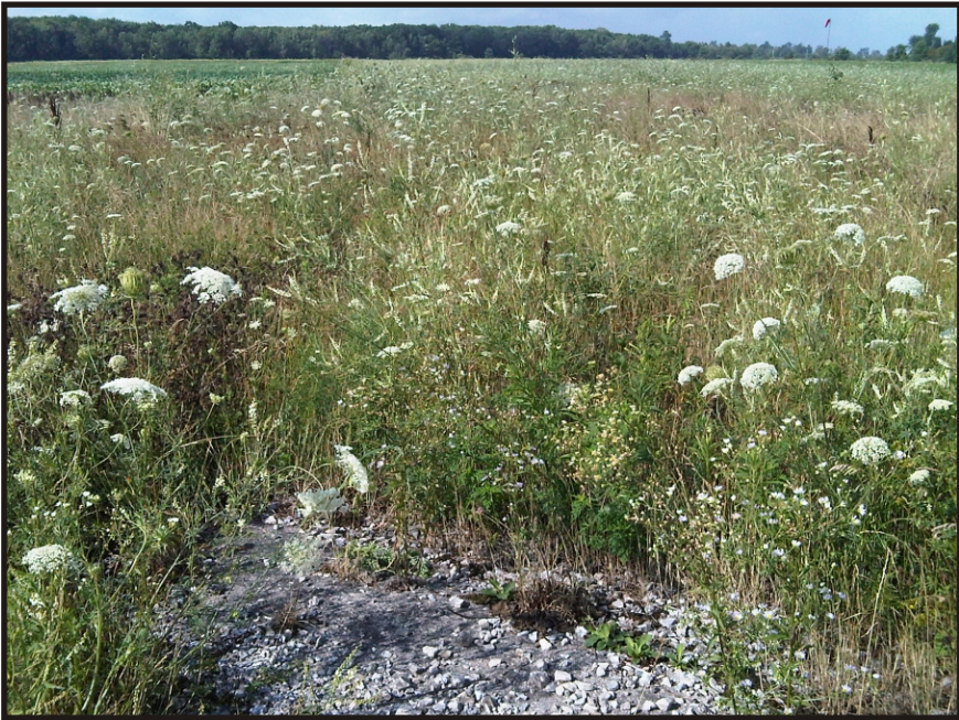
Photo 11 - Concrete Under Weeds In Infield of Runways
