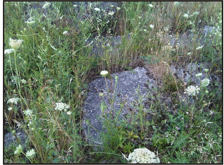
Photo 10 - Decaying Asphalt of Old Runway Under Weeds, South of Access Road for Turbine 61
