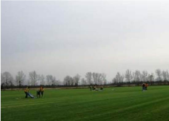
Photograph 91: View of AMEC personnel conducting test-pitting program within Parcel 14A, facing southwest.
