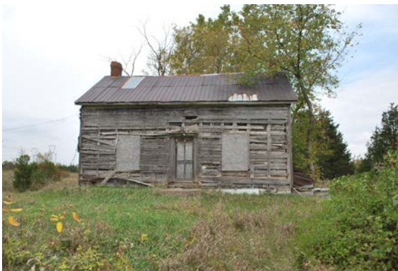
View looking north from Unity Road at front façade of derelict farmhouse.
