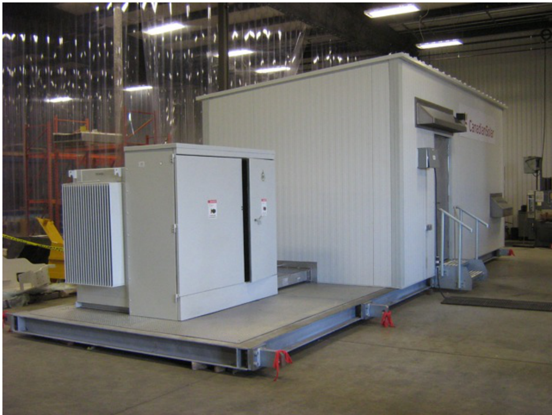
Photo: 1.6 MVA eHouse with intake and exhaust rain hoods but no silencers
