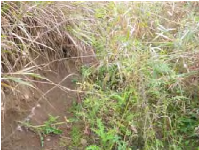
Photo 3: Erosion upstream from Rock Rd. culvert. Site ID# P1-A
