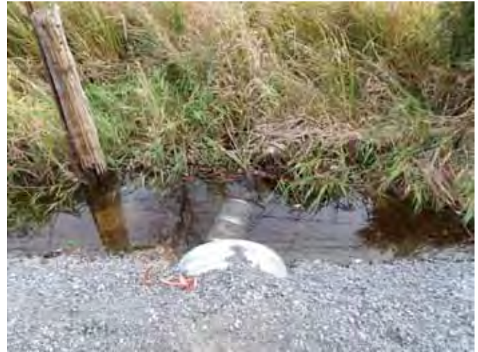
Photo 106: Looking south at intermittent drainage with water at roadside ditch. Site ID# SP18-D
