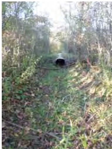
Photo 87: Continuing to look west at drainage swale/lane where culvert has been placed to maintain lane crossing. Site ID# P23-Northern-1
