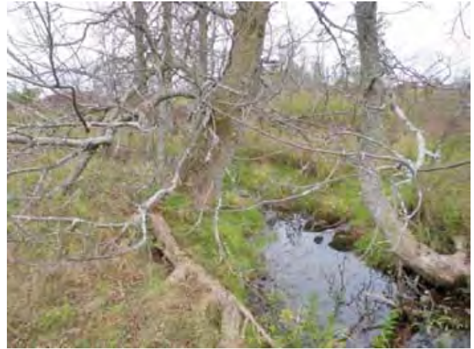
Photo 46: Looking north just upstream from box culvert. Wetted depth is ~0.18m. Site ID# P6A-A
