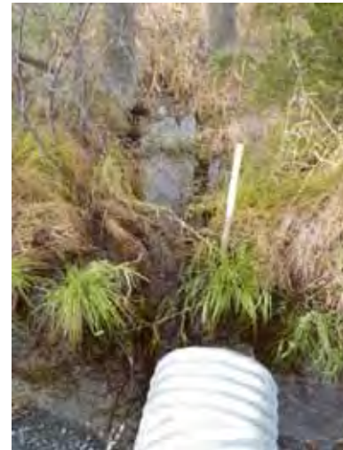
Photo 108: Channel width wetted is 0.85m, with a substrate of silt and limestone. Site ID# SP18-D
