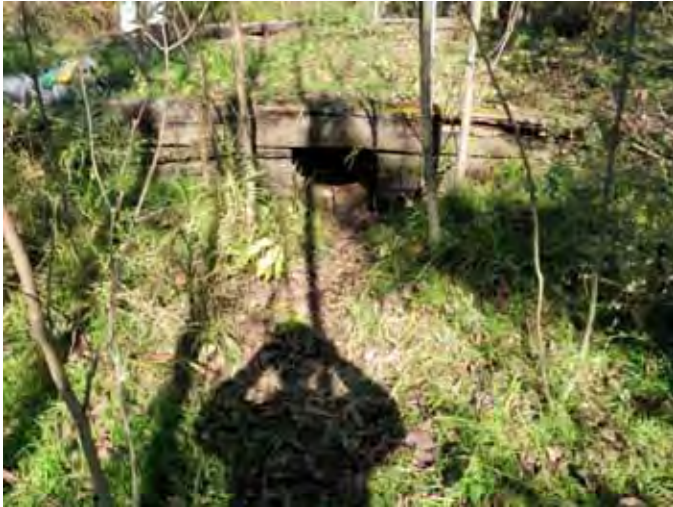
Photo 69: Looking north, CSP and cradle structure at the end of an access laneway near the Flying J billboard. Site ID# P24-B
