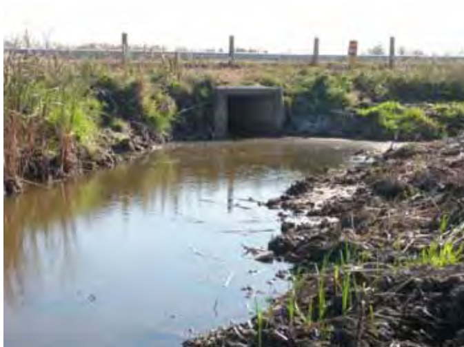
Photo 67: Highway 401 box culvert crossing at ROW, 6mx8.5m pond. (Millhaven Cr. Trib.1) Site ID# P24-A
