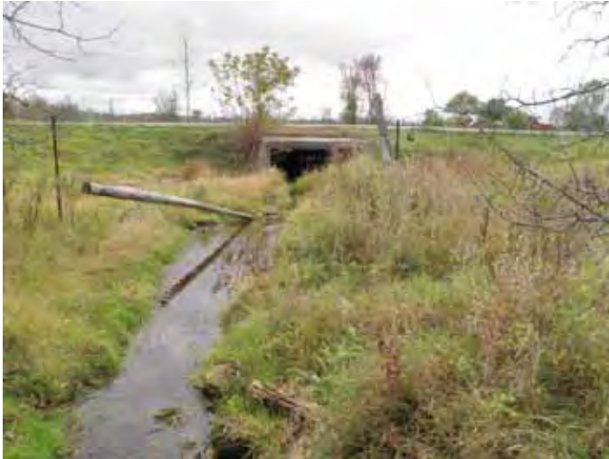
Photo 45: Looking south at box culvert at Unity Rd. crossing. Flow is downstream into P14B pond. Site ID# P6A-A
