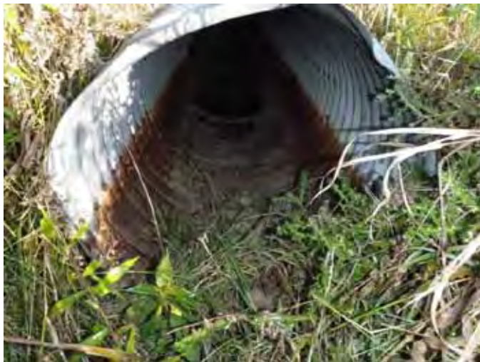
Photo 83: Looking into dry CSP on south side of Mud Lake Rd. Scour at mouth indicates water conveyance with roadside ditch during wet periods. Site ID# OL-A
