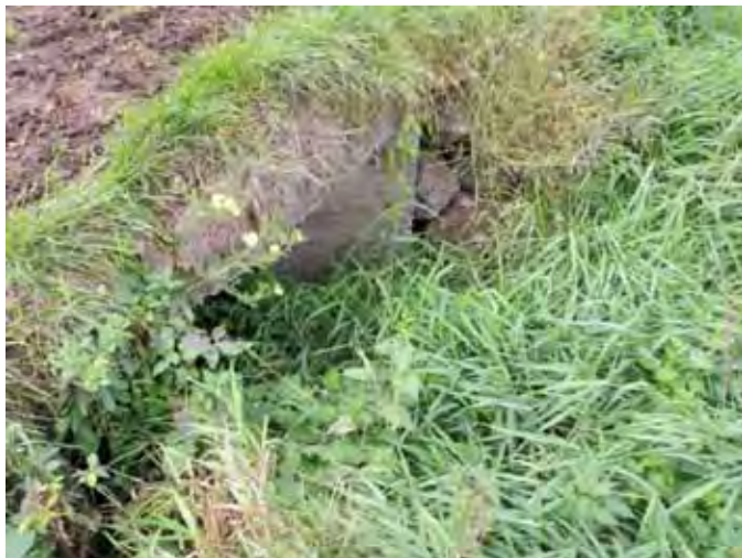
Photo 39: Glenvale Cr. Trib.2c culvert has standing water in depression and is choked with vegetation. It's suspected to be an intermittent swale. Site ID# P6A-2
