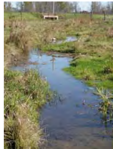
Photo 92: Looking north at box culvert crossing at Unity Rd in cow pasture area upstream of man-made Property 14B Pond. Site ID# P14-B2
