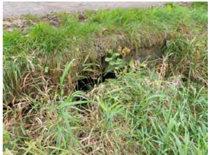
Photo 40: Pool from culvert on east side of roadway choked with vegetation. No channel or swale observed. Site ID# P6A-2
