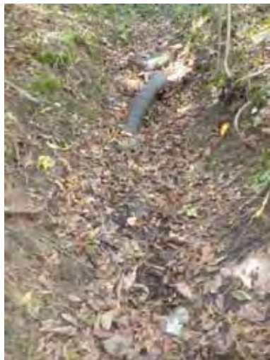
Photo 63: Upstream of P20-B2 a corrugated plastic pipe was found exposed in the channel. Channel leads to base of cleared field that likely drains to this feature. Site ID# P20-B2
